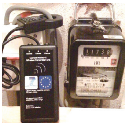
Figure 1 – Clamp transmitter (current transformer sensor)
