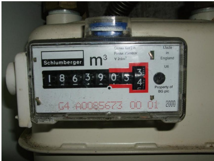
Figure 14 Gas Meter Display
