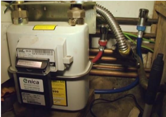
Figure 6 Dehems Equipment – OCR Gas Reader
