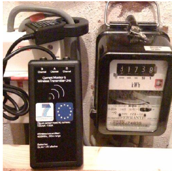
Figure 5 Dehems Equipment - Installation at the Meter
